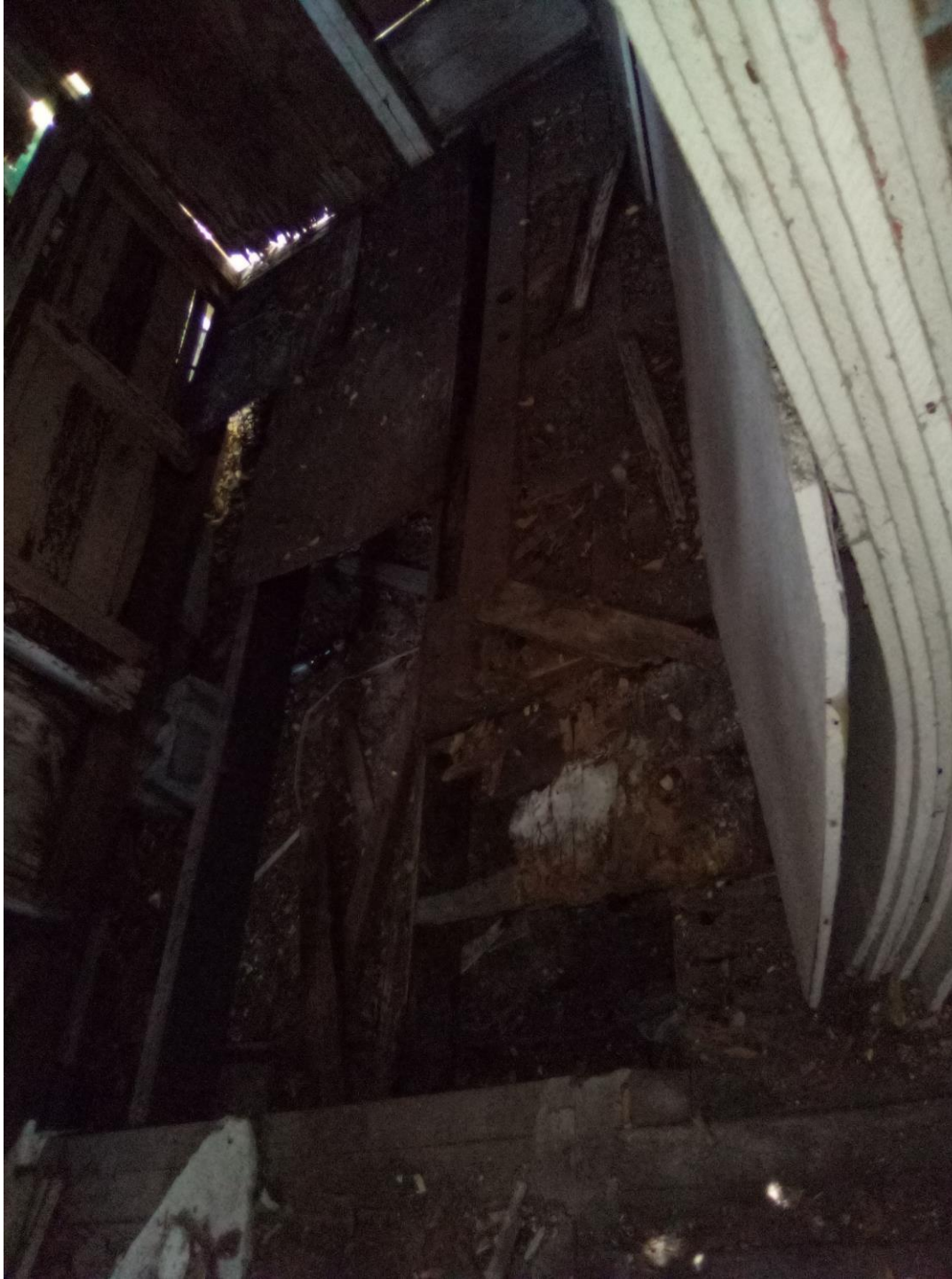
Rotted and Settled Floor
