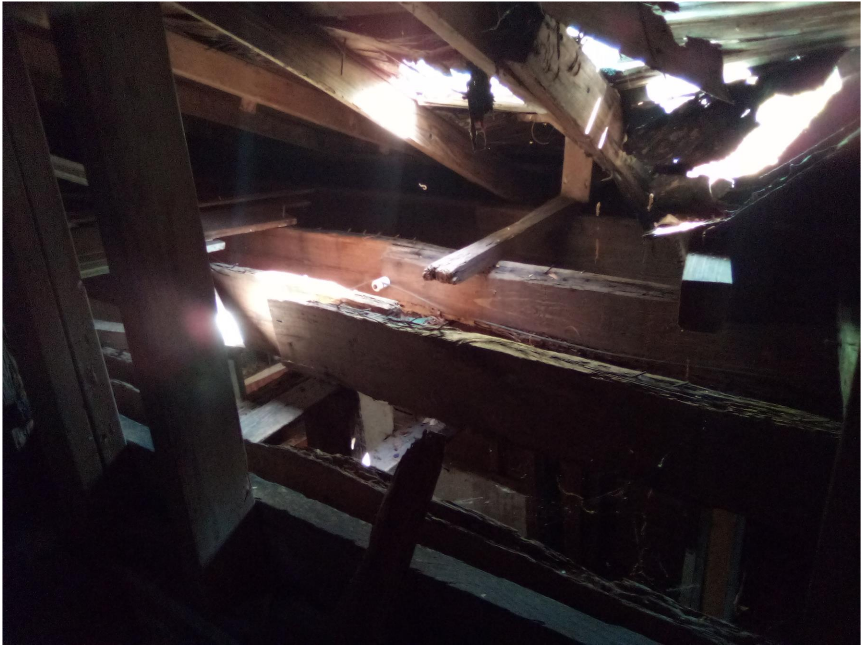
Rotted Trusses and Roof
