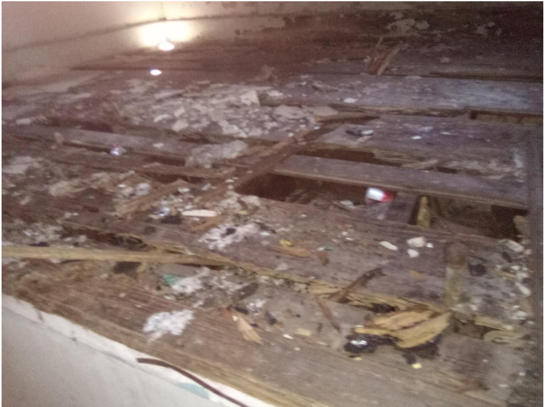
Settled and Rotted Floor
