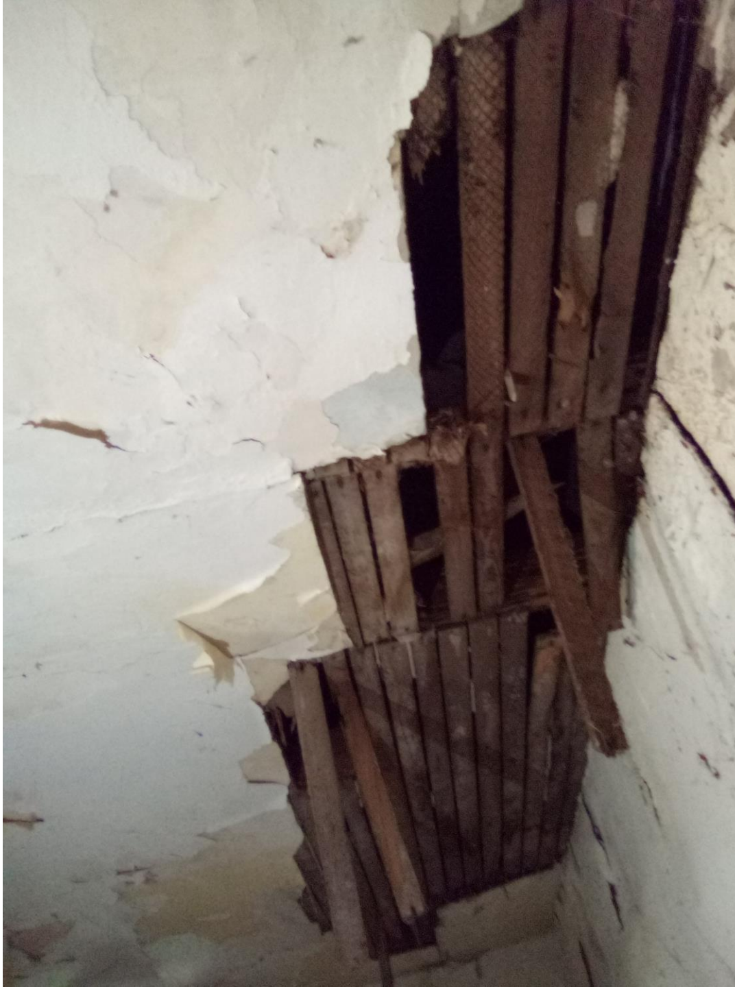
Ceiling Damage From Water Intrusion
