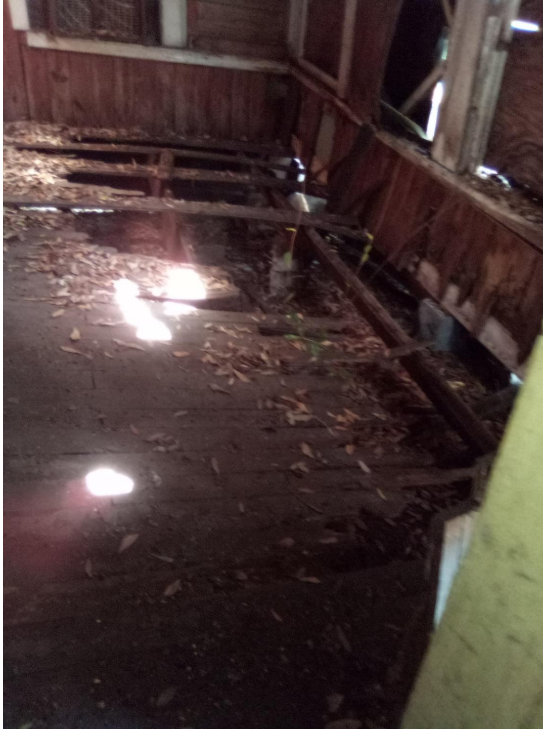
Floor and Joist Damage and Settling
