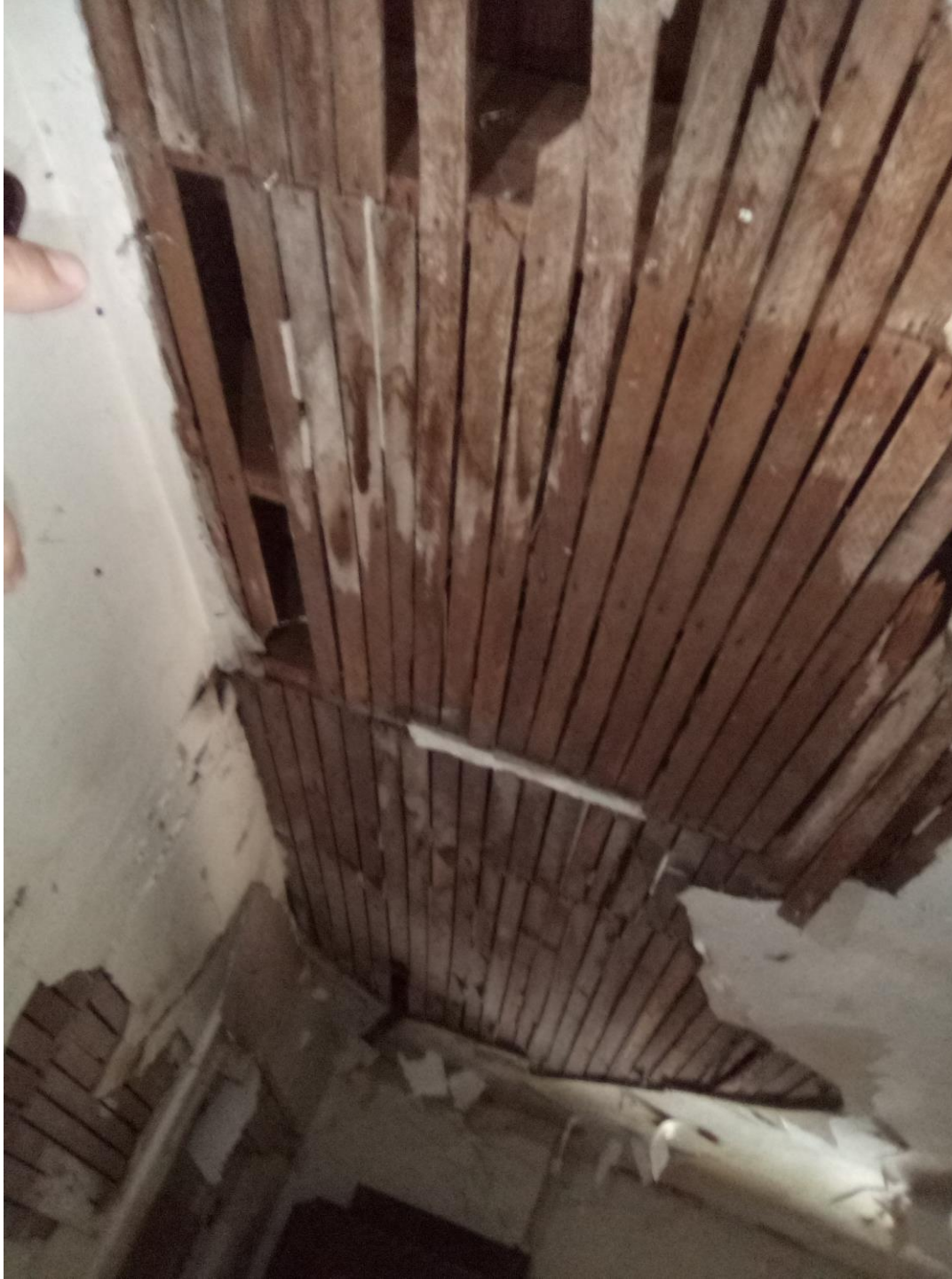
Ceiling Damage From Water Intrusion
