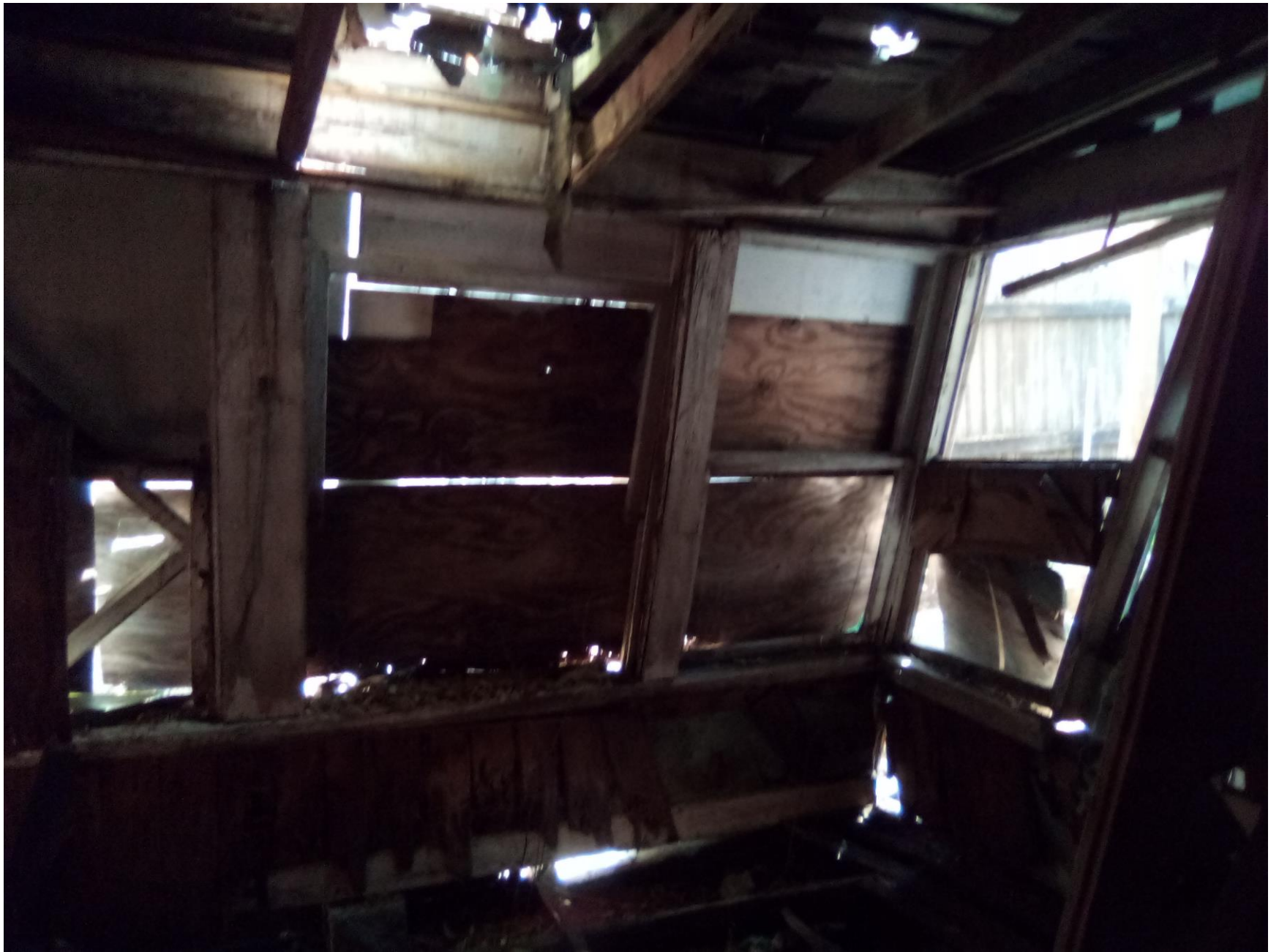
Rotted Roof, Wall, and Window
