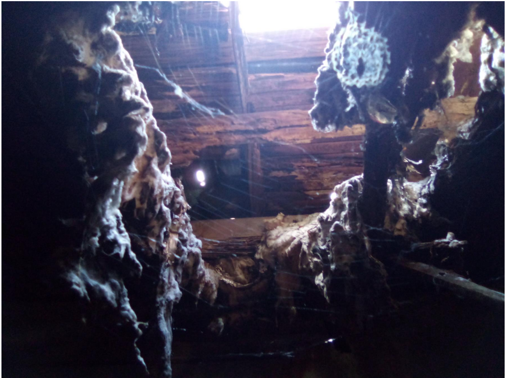
Upstairs Ceiling, Rotted Trusses, and Water Intrusion
